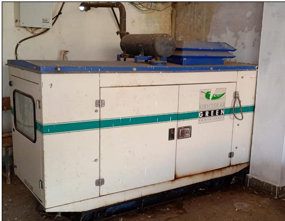
Figure 2.1:- DG set on the college campus
